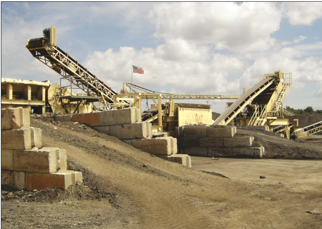
The STS 2618VM stationary screening plant from Astec Mobile Screens may be hard to spot in these photos of the Banks Construction Company plant site—but it is a key element in their effort to fractionate RAP to help them achieve high production rates while maintaining their tight quality-control standards. The STS 2618VM screens the RAP material into two sizes. The company maintains stockpiles of about 4,000 tons (3,600 tonnes) of each size of RAP.
