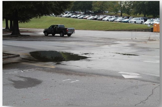
"Bird bath" due to inadequate pavement slope.
